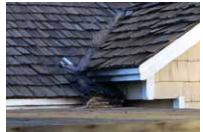
Reducing the structural ignitability of houses, such as replacing wood shake roofs and removing pine needles, is a CWPP objective.
