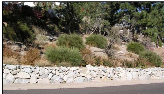
Figure 3. The eroding hillside in the upper photo has greater than a 50 percent slope. It is easier to grow plants when a retaining wall holds up the toe of the slope, as shown in the lower photo.
