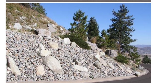
Figure 4. Retaining walls (top) and rock slope protection or rip rap (bottom) prevent erosion on steep slopes.
