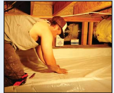
Kaleb Ennis lays out the polyethylene sheeting over the dirt in the crawl space.
