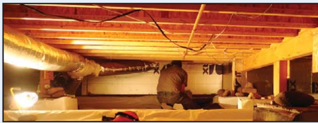
A mitigation crew member adheres the polyethylene sheeting to the stem walls and floor joists in the crawl space.
