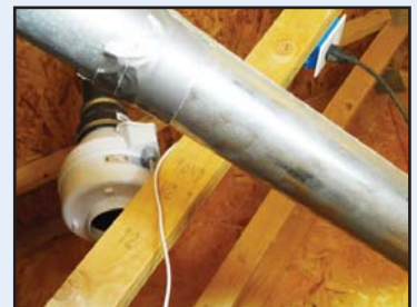
A radon fan was installed in the attic, along with as an electrical outlet to power the fan.
