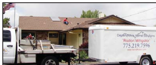
Derrick Carpenter works on the White's rooftop, installing the vent pipe for the radon mitigation system.
