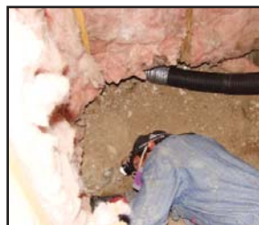
Carpenter drills through the foundation to connect the pipe from the crawl space to the fan in the attic at the White's home.
