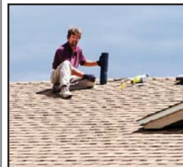
Derrick Carpenter is pictured on the roof at the Doyle's home, installing the pipe that will exhaust radon gas out from beneath the home to the atmosphere. The fan is located in the attic area and pulls air from under the home.
