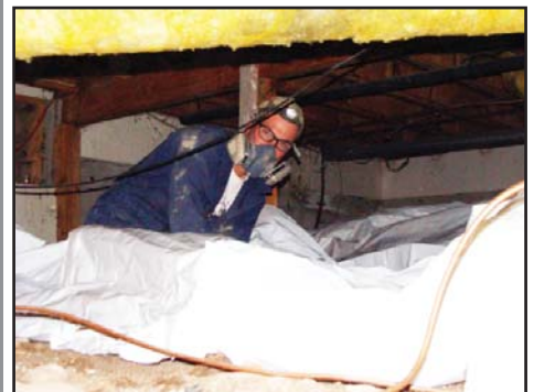
Eric Class assisted Carpenter in laying the poly sheeting in the crawl space at the White's home.
