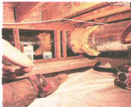
UNIVERSITY OF NEVADA COOPERATIVE EXTENSION A mitigator caulks the crawl space sheeting.
